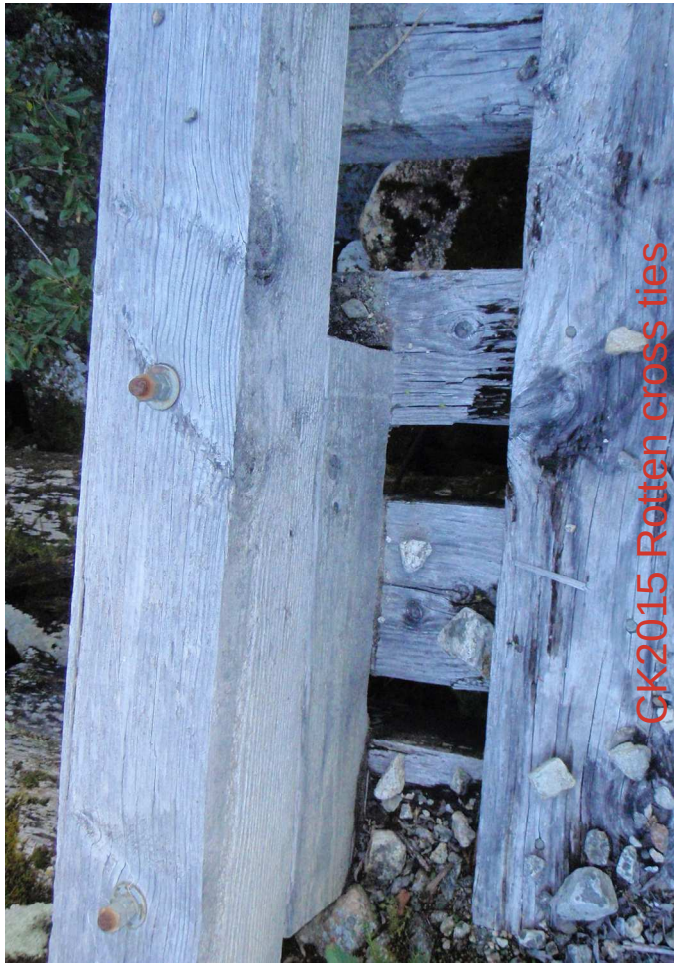
CK2015 Damaged rail
